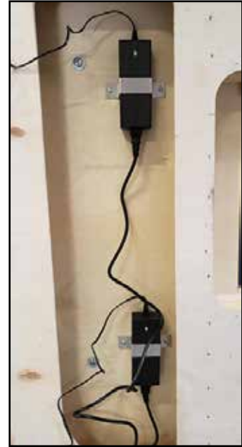
Transformers on back of panel
